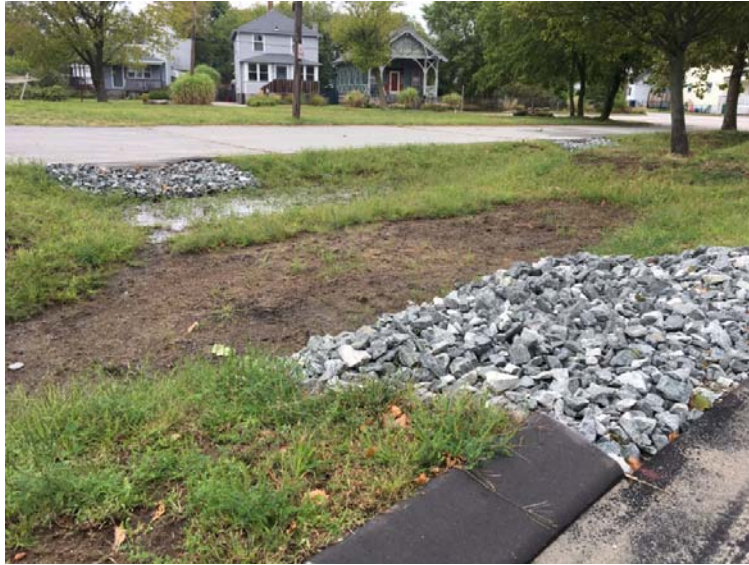
Figure 2. Bio-Retention basin with bio-retention media and stone erosion controls.
