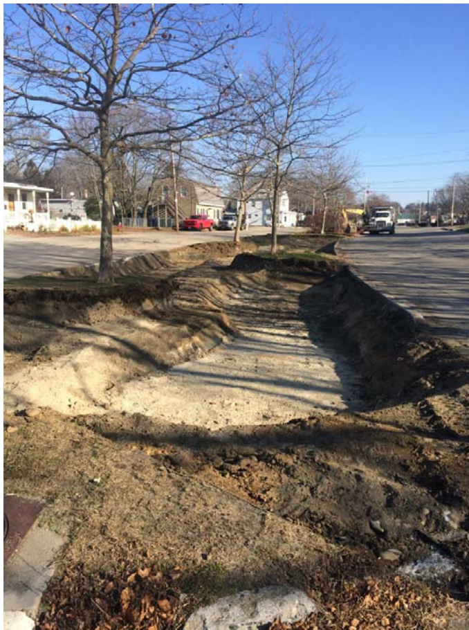
Figure 1. This photo shows one of the bioretention locations with top soil removed and rough grading to sub grade material.
