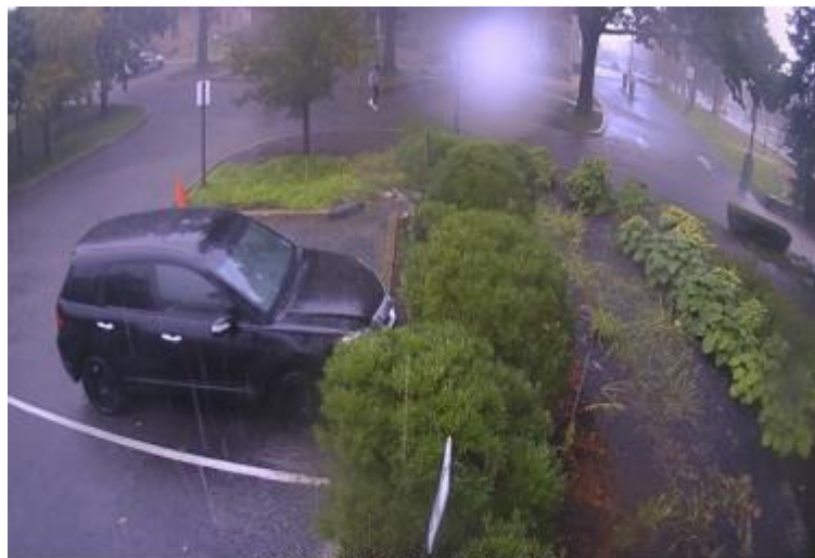
Infiltration basin treating runoff from parking lot at Providence College during heavy rain event. Inlet is working and berms are mostly containing flows. Overflow bypass appears to be functioning as intended. Photo: ASRI.
