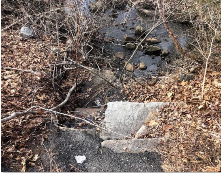
A paved swale directing untreated runoff to highly degraded section of the unnamed tributary to the Runnins River. Photo: East Providence, Rhode Island.
