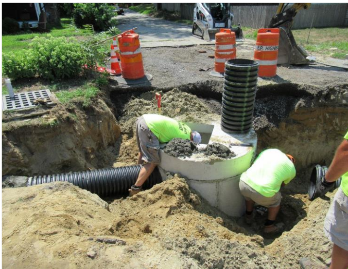
Retrofit installation on Willow Street in East Providence, Rhode Island. Photo Credit: East Providence, Rhode Island .
